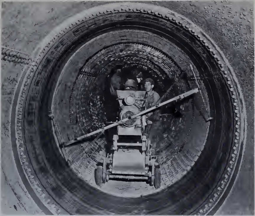
Figure 206.—Trowels smoothing mortar which has been spun to the pipe surface by the rotary head in the lining machine. This produces a surface which has good hydraulic flow characteristics. P126-100-18.
